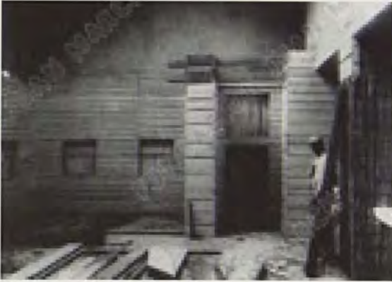
Left side-hall of the Secession Building during construction work for the Beethoven Exhibition, 1901
